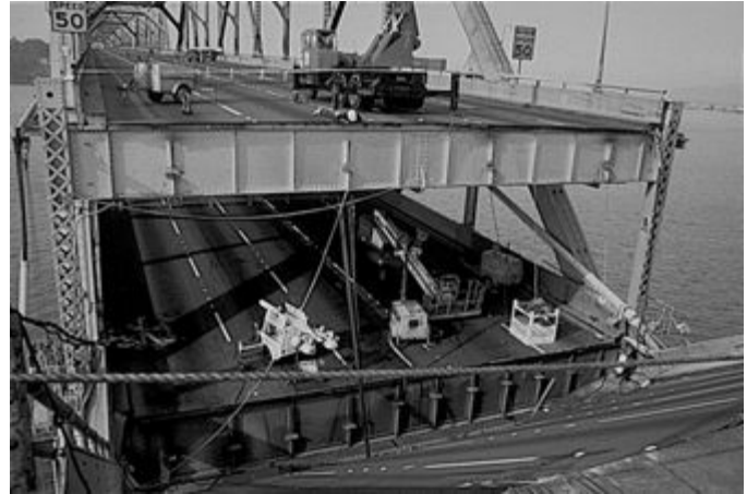
Fig. 1.2-8 Damage to the Bay Bridge, connecting San Francisco and Oakland, from the October 17, 1989, Loma Prieta earthquake. The bridge is of old construction (1936), and its supports rest in sedimentary fill that amplifies ground shaking. (Courtesy of the US Geological Survey.)
